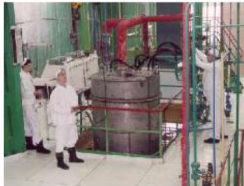
PROTOTYPE DEMONSTRATION PLANT CATALYTIC REACTOR (SECOND FLOOR VIEW (NOVOSIBIRSK))
